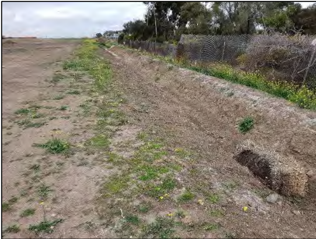
Plate 15. Drainage line constructed on the southern boundary of the study area looking east (Ecology and Heritage Partners Pty Ltd 07/09/2018).
